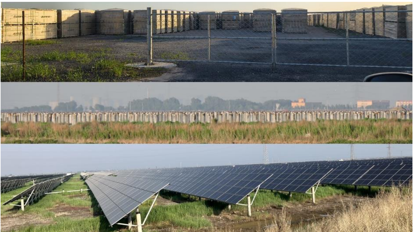
New panels sacked and ready to go on to concrete posts to harness the sun
